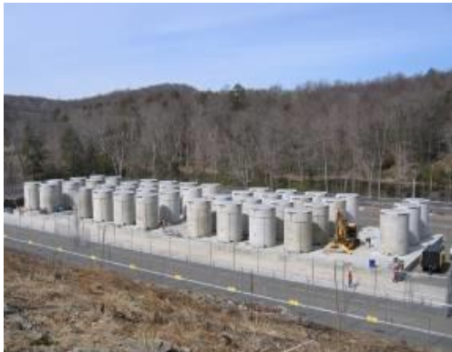
The Independent Spent Fuel Storage Installation (ISFSI) Maine Yankee NPP (USA)
